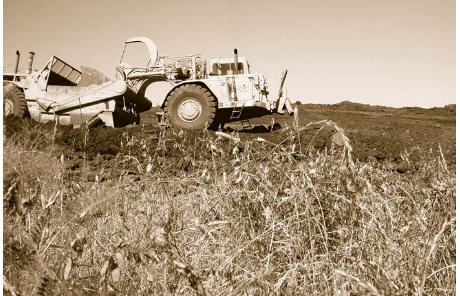
Bulldozers created the contours of the berms at the Green Music Center site. Construction equipment will return to the site this spring to begin building the center.
